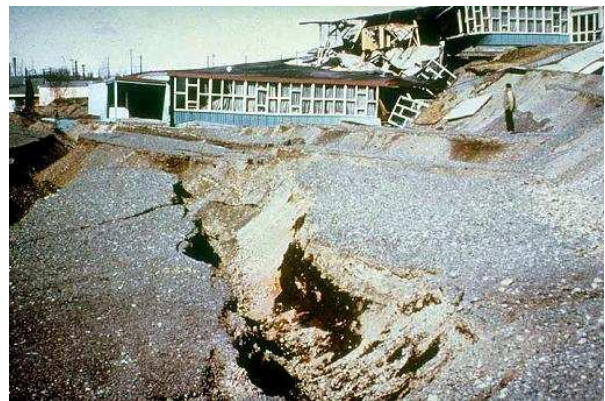
Government Hill Elementary School torn apart by subsidence that occurred during the 1964 earthquake. Notice the large crack in the foreground that also was caused by the earthquake, (9.2 magnitude).
